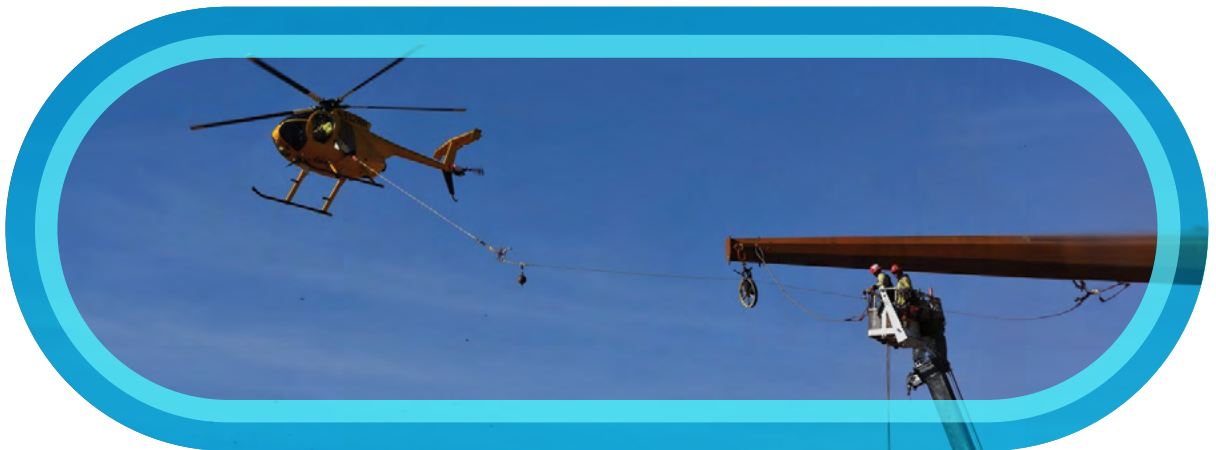
David McColl, Winco utility helicopter pilot and director of safety and training, flies an MD 369FF in support of power-line construction and maintenance.
