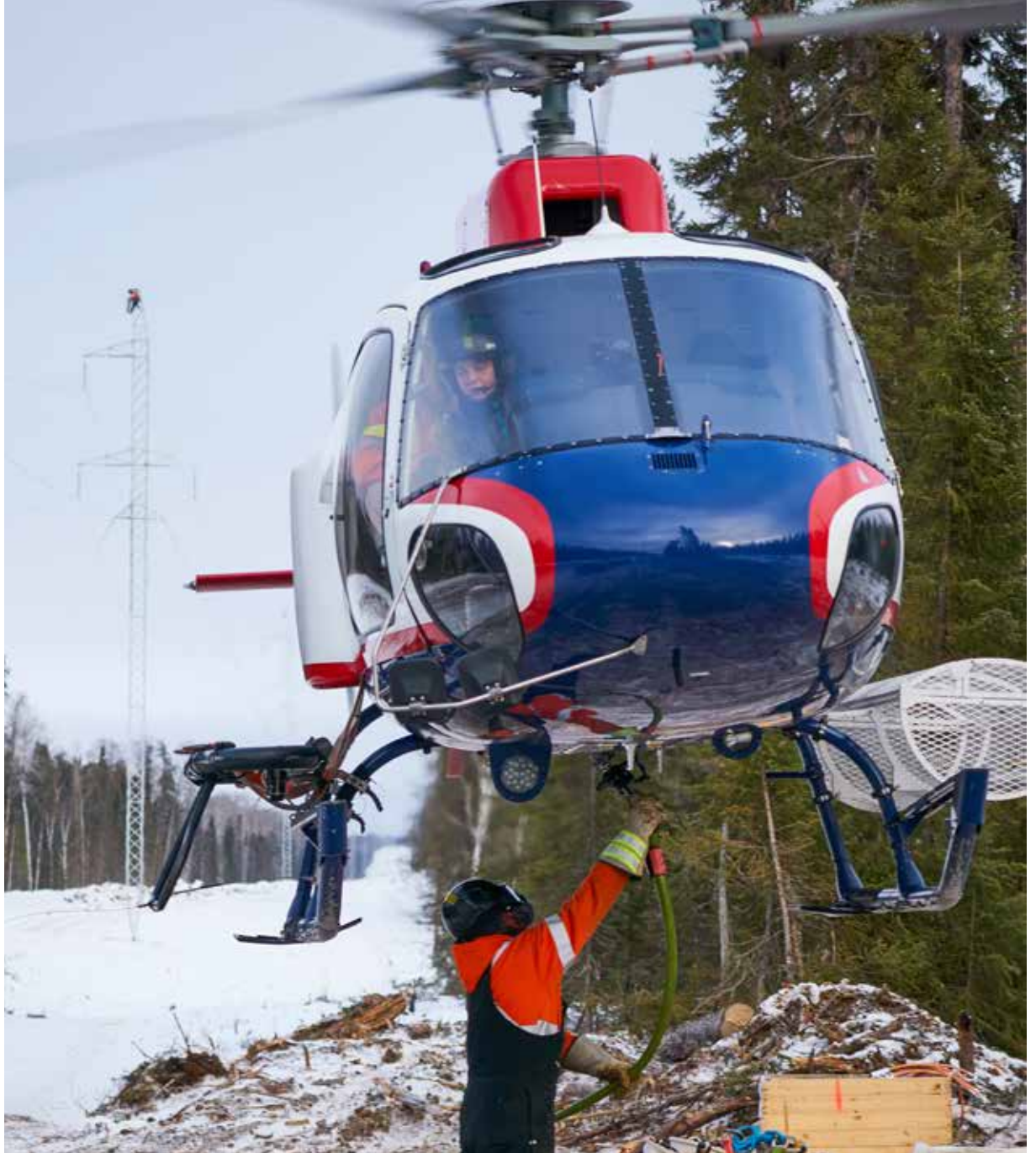
Type 3 helicopters, such as this AS350 B3, perform myriad jobs on utility projects, including carrying sling loads from staging areas.
