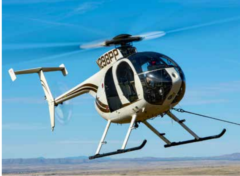
Near Belen, New Mexico, an MD Helicopters MD 500E operated by Rotor Power pulls a sock line during construction of a line of transmission towers.
